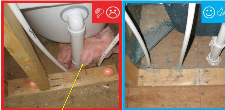
Courtesy of the Department of Energy's Building America Solution Center ( http://bascc.energy.gov )
