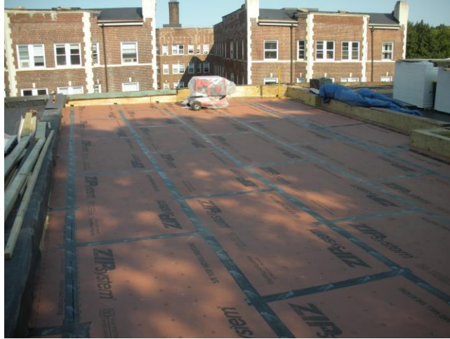
Courtesy of the Department of Energy's Building America Solution Center ( http://bascc.energy.gov )
