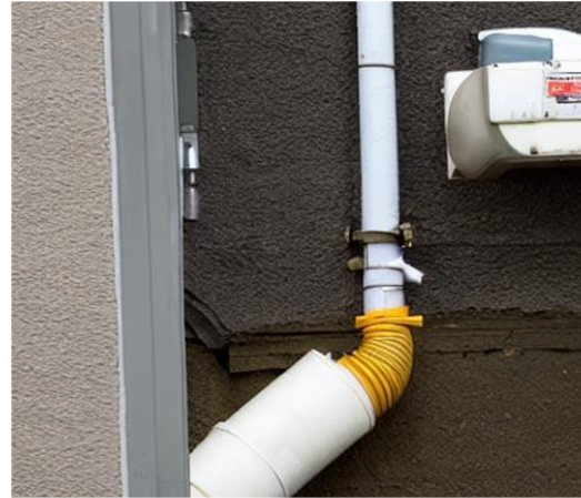
BTM Gas Leaks
